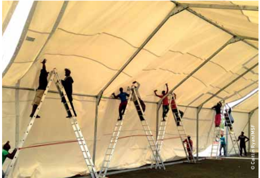
Monrovia, Liberia. Construction teams building what would become ELWA 3, the world’s largest Ebola management centre with 250 beds.
